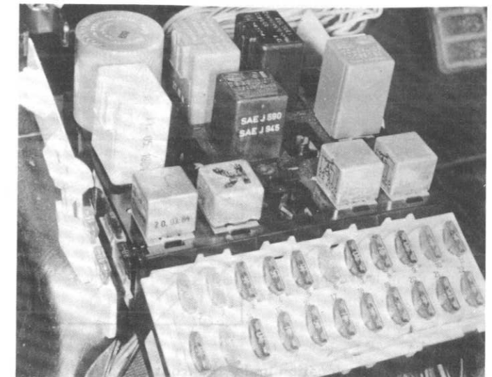
24.4B ... and withdraw the central electrical unit. (Centre console has been removed)
