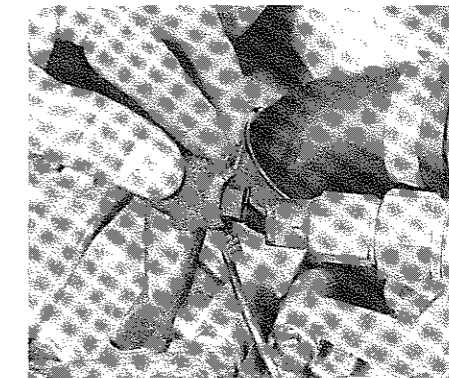
34.30 Disconnecting the thermal timer multi-plug
