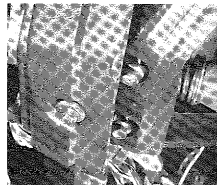
13.8 The three bolts which secure the column top bearing to the crossmember
